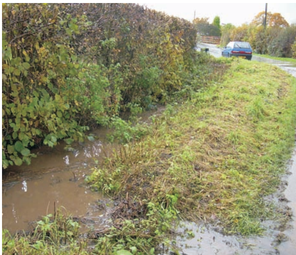
Roadside drainage needs to be maintained
