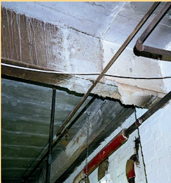
Sprayed Asbestos and Lagging.
