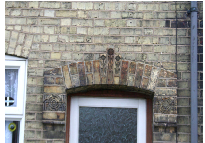
6. Fine brick detailing on a Victorian window in the Historic High Density Zone.
