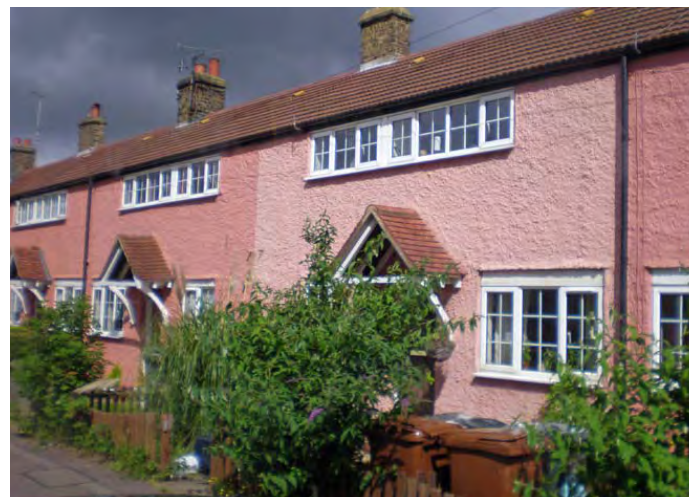
3. Pink painted render and UPVC windows dilute the distinctive Garden City character.
