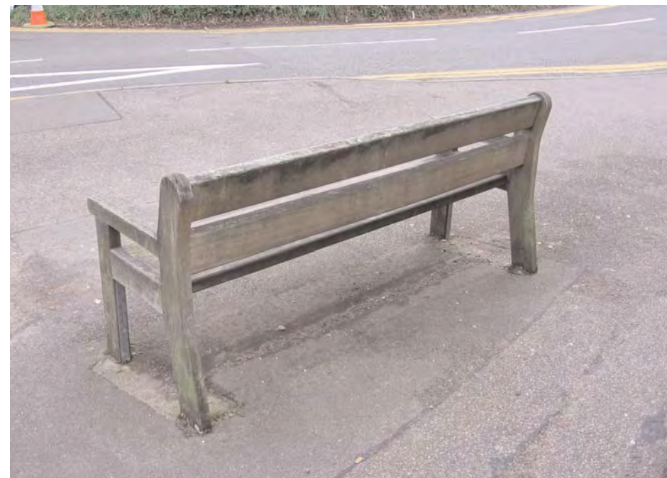
3. Items of street furniture are well utilised, but could benefit from a coherent strategy aimed at enhancing aesthetic appeal and maintenance.
