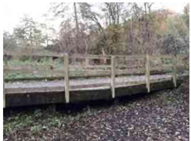
Bowed boardwalk structure
