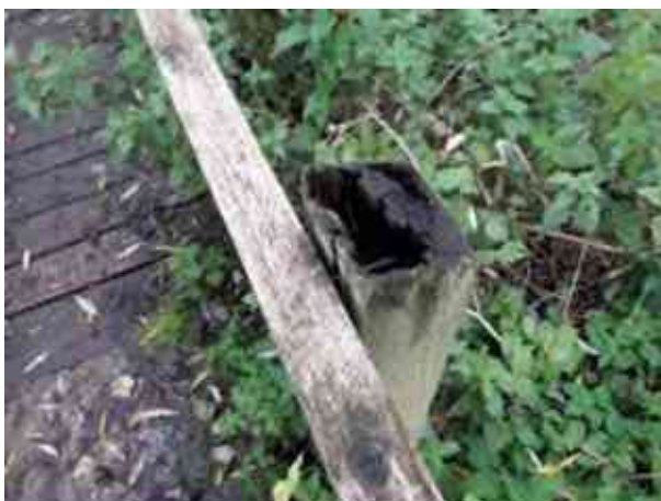
Rotten post on boardwalk
