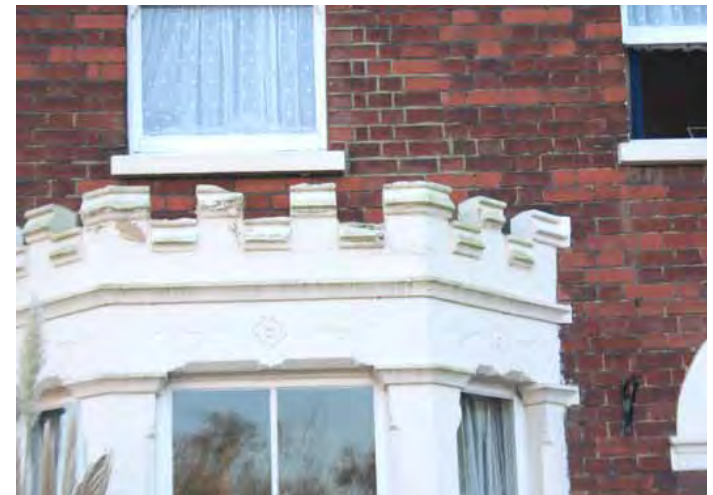
4. A Victorian house on Baliol Road; red brick with a white castellated bay window.
