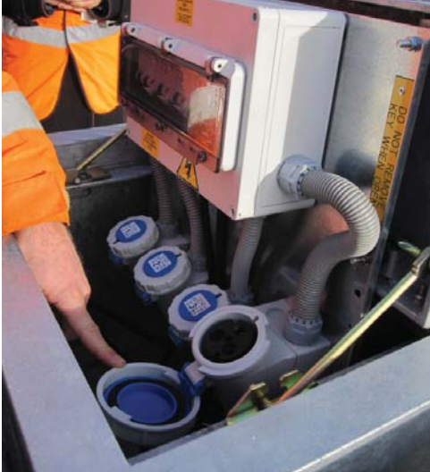
In ground power supplies
