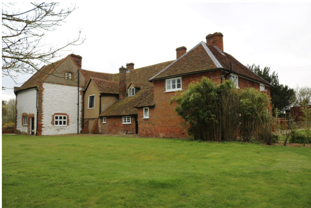
Plate 4: View of the rear (north) elevation of the house showing the sweeping 'catslide' clay tiled roof, and a projecting roughcast rendered timber-framed staircase wing
