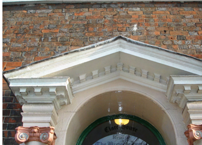
1. Elegantly decorated eaves supporting a projected first floor, common among timber framed houses in the Town Centre zone.
