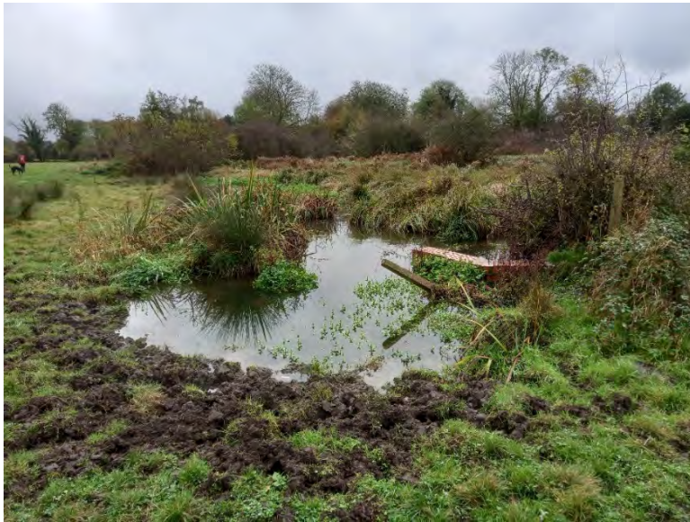
Poached area around culvert outfall into the river channel
